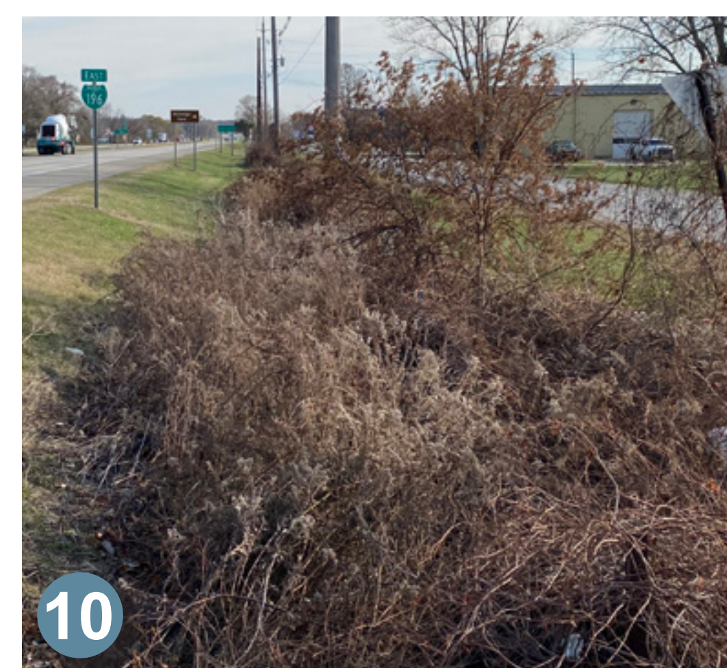
10 Drainage ditch between roads has vines and weeds that collect trash.
