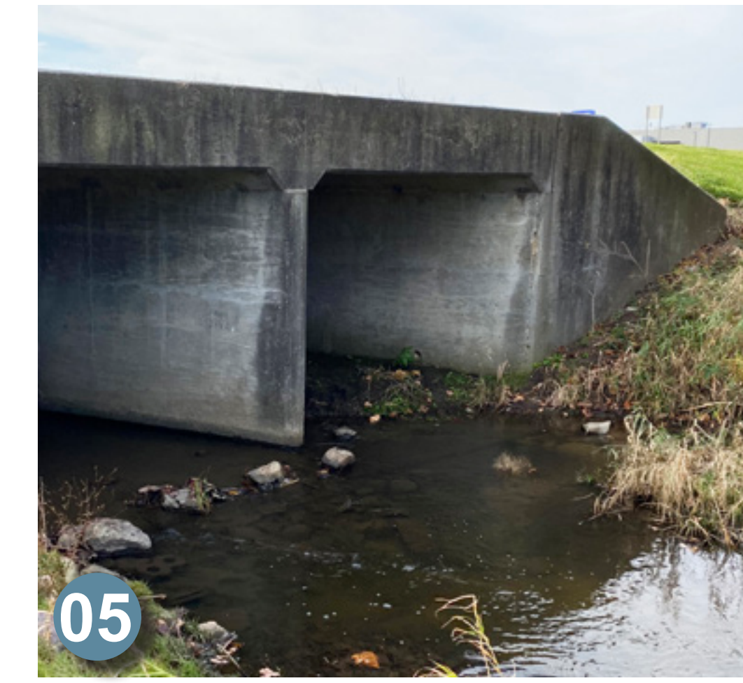
05 Box culvert allows drainage under the road.
