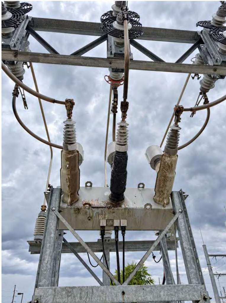
Lightning Damage to FV-6 Recloser
